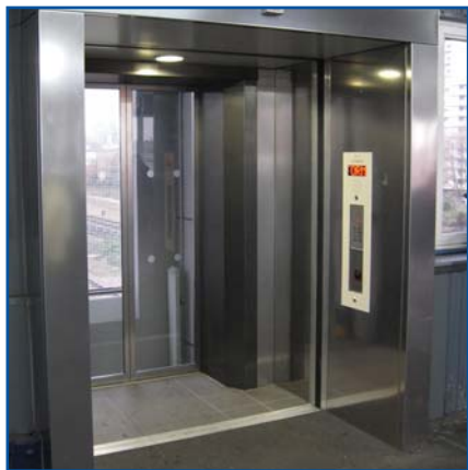
New lifts at Clapham Junction.
